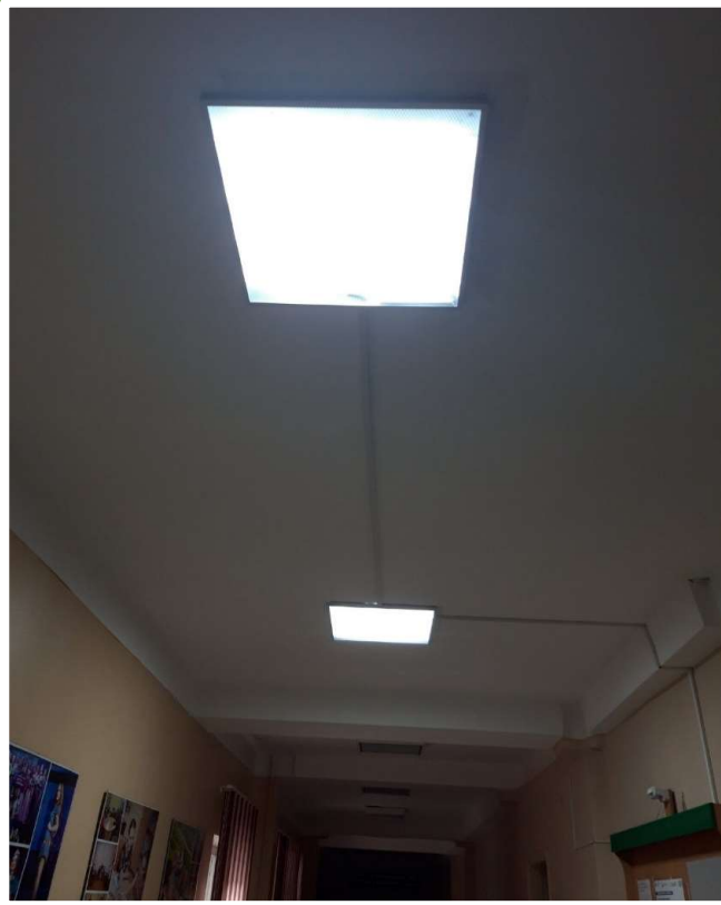
Energy saving light bulbs with motion sensor
